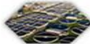
Waste Water Treatment
